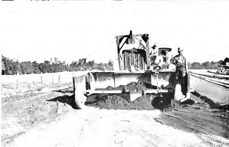
At top—Truck dumping cement stabilized mix in bulldozer spreader box. Below—Bulldozer equipped with forward steel wings attached to ends of blade and wheels spreading mixture approximately 14 inches deep on roadway
